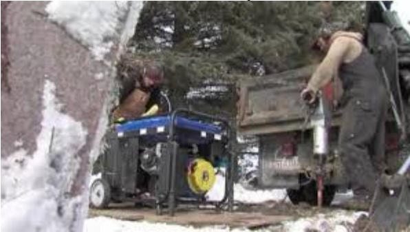
Brothers Matt and Andrew Goeden dig graves with jackhammers and backhoes in Henning, Minn. Photo courtesy of CNN.
