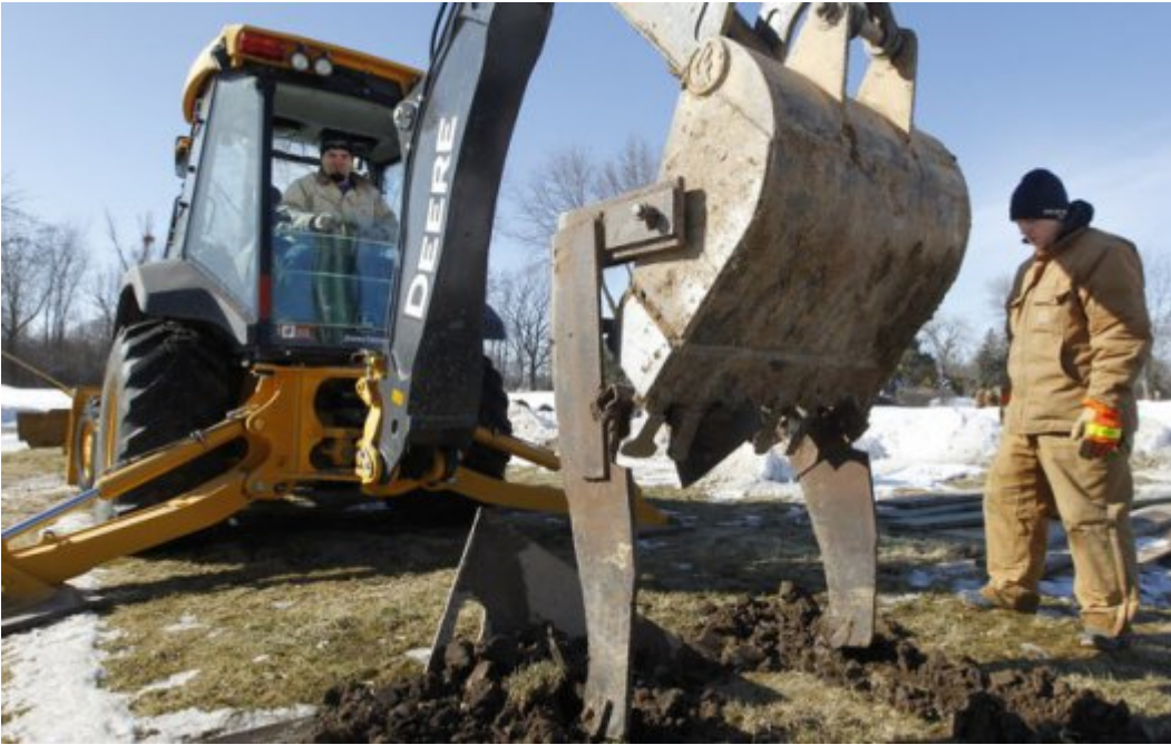
Cory Lidwin (left) and Rick Budnick use “frost teeth” attached to a backhoe while digging a grave at Highland Memorial Park Cemetery in New Berlin, Wis. Photo by Mark Hoffman, Milwaukee Wisconsin Journal Sentinel .
